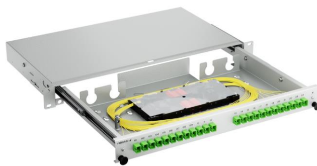
Example of equipped patch panel
